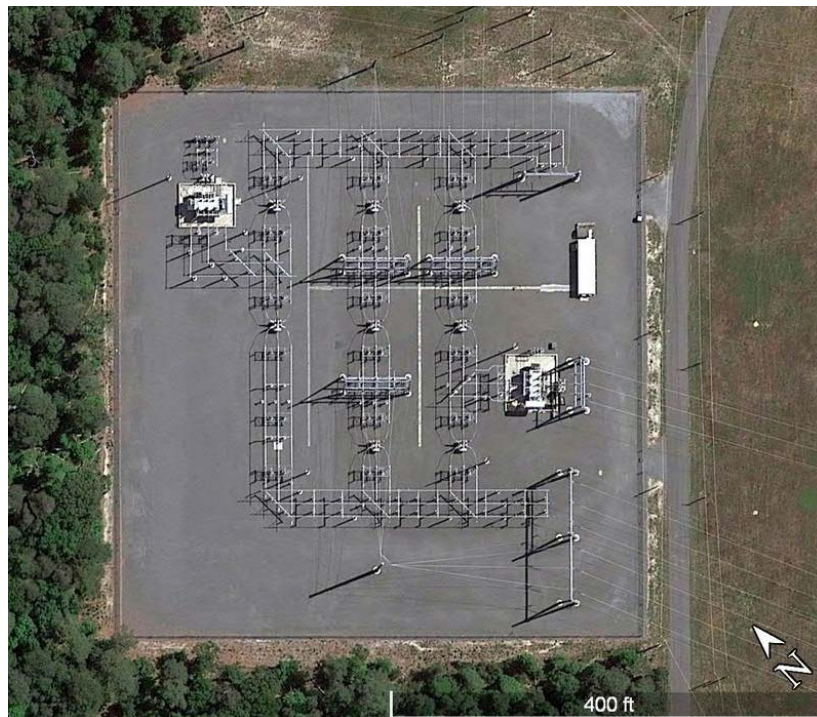
Figure 2-19. Indian River Substation
